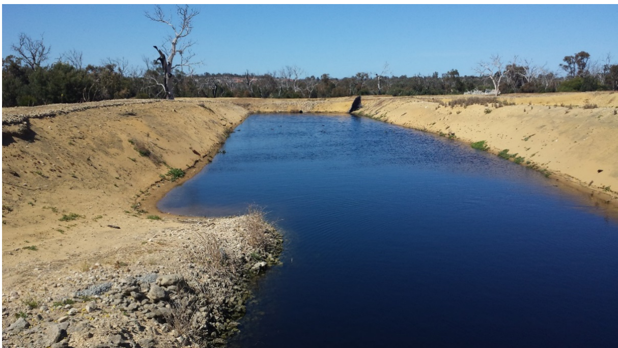
Example of an infiltration basin, located at the Kwinana wastewater treatment plant (2016)
