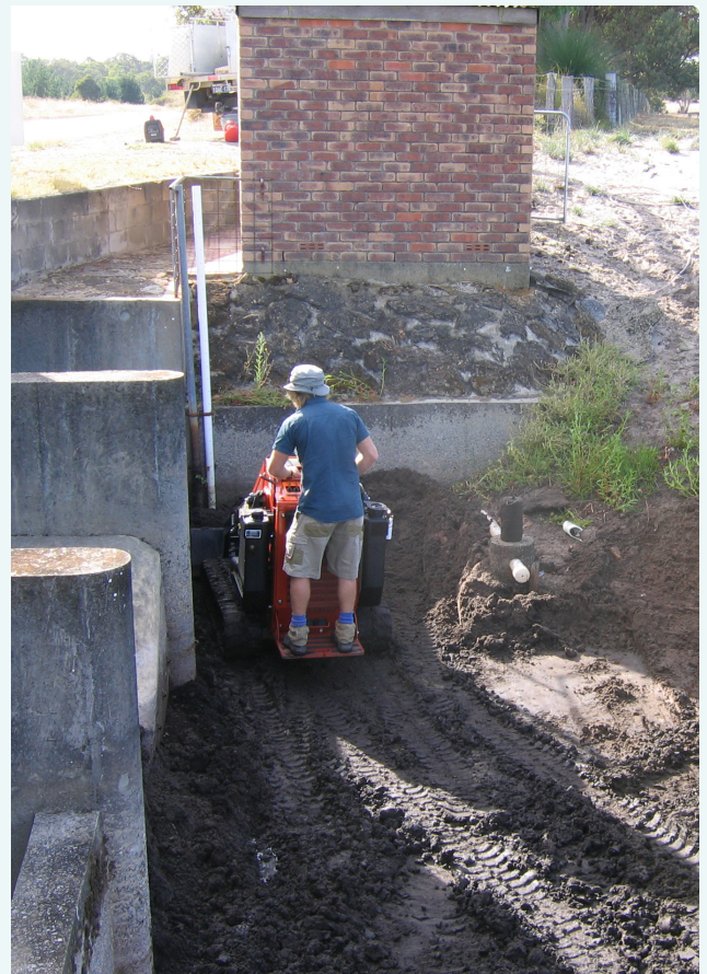
Removing particulate matter and sediments which have settled in front of the gauging station at Meredith Drain, May 2020.
