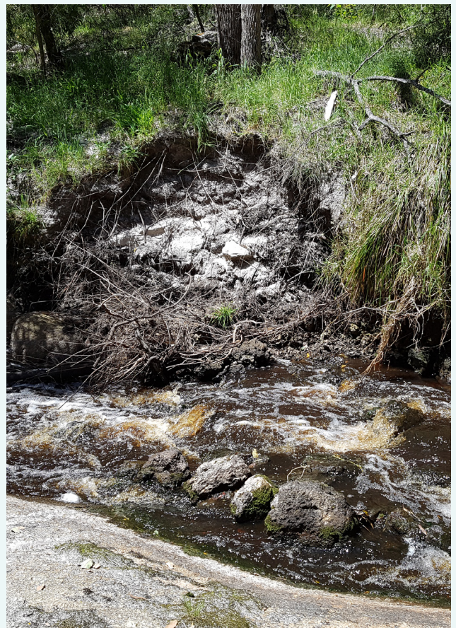
Undercutting of the bank near the sampling site has caused it to slump, October 2017.
