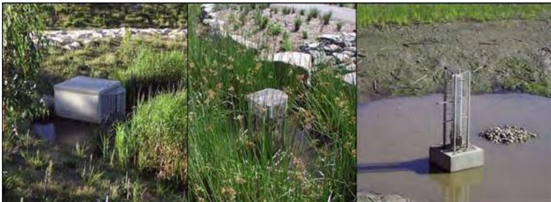
Figure 6. Debris guard examples for riser outlets. (Source: Morton Bay Waterways and Catchments Partnership 2006.)
