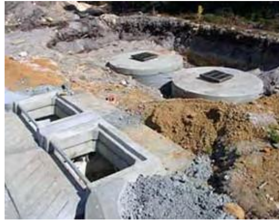
Figure 6. Construction of side entry pits to capture road runoff and divert it into soakwells that have bubble-up lids and are located within a detention area. (Photograph: TME 2003.)
