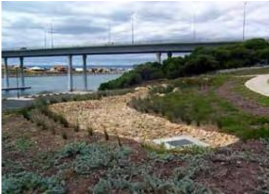
Figure 1. Bioretention swale, soon after construction and planting in Dawesville. (Photograph: Grahame Heal, City of Mandurah, 2006.)
