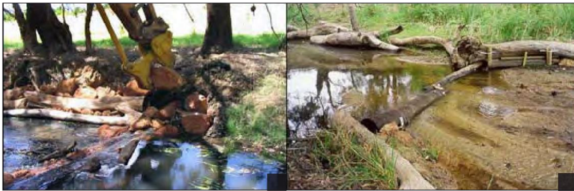
Figure 5. a) Construction of a log and rock riffle structure in the Canning River, Pioneer Park, Gosnells. (Photograph: Department of Water 2004.) b) Log riffle built on the South Dandalup River, Pinjarra, to stabilise the sandy riverbed, induce a scour pool and enhance habitat diversity. (Photograph: Water and Rivers Commission 1999.)
