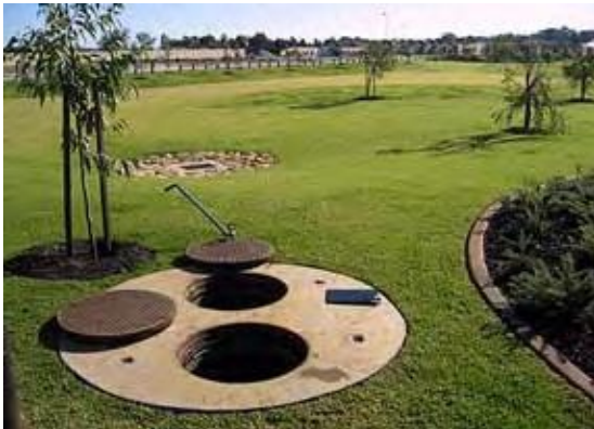
Underground chamber device GPT, Backshall Place, Wanneroo. (Photograph: JDA Consultant Hydrologists 2004.)
