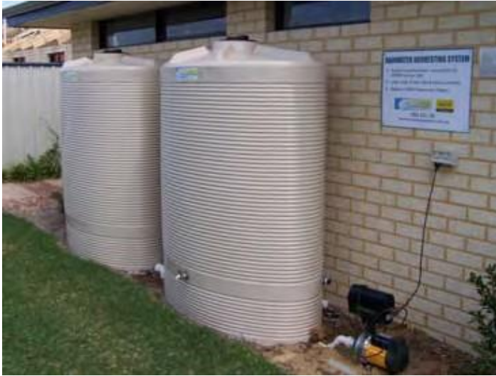
Demonstration domestic rainwater tank. (Photograph: Renee Romyn.)
