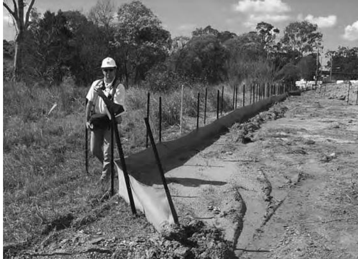
Figure 5. Silt fence for controlling sediment during land development. (Photograph: André Taylor, Ecological Engineering Pty Ltd.)
