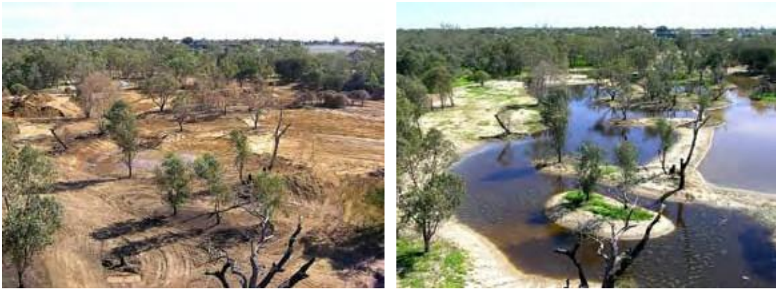
Liege Street Wetland, Cannington, during construction in May 2004 and immediately following completion of construction and initial planting in September 2004. (Photographs: Department of Water.)
