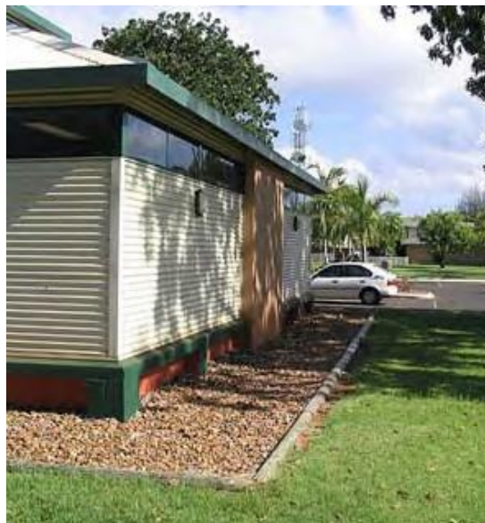
Pervious surface under gutterless roof, Shire of Broome. (Photograph: Allan Ralph, Shire of Broome 2005.)
