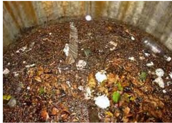
GPT chamber following a storm event, near Lake Jualbup, Shenton Park. (Photograph: JDA Consultant Hydrologists 2005.)
