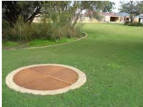
Figure 3. Bubble-up pit located in a park. (Photograph: Department of Water 2006.)
