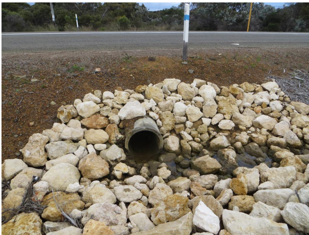
Figure D6 Stormwater drainage in Bremer Bay
