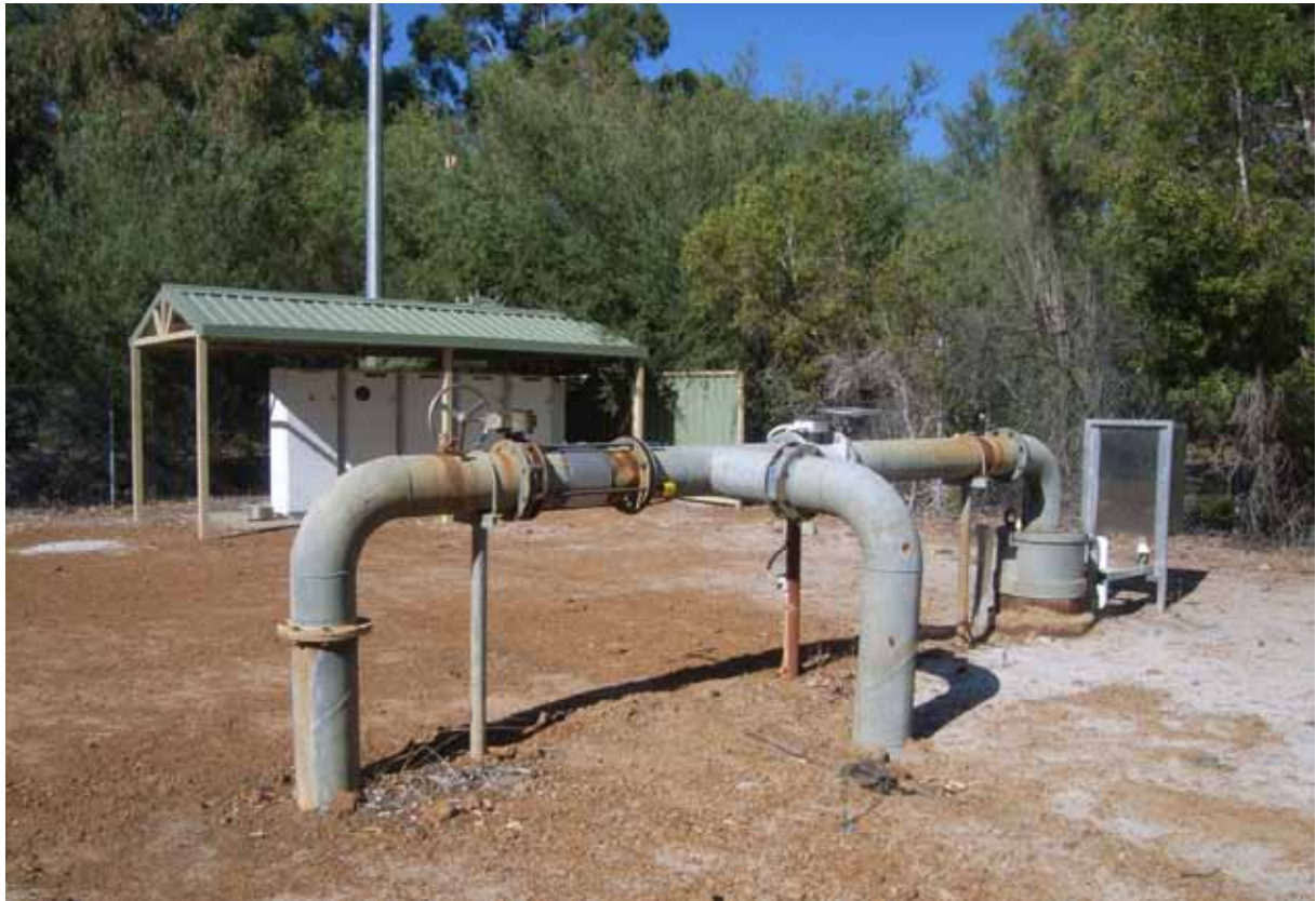
Figure C3 Australind Water Reserve production bore 3/92
