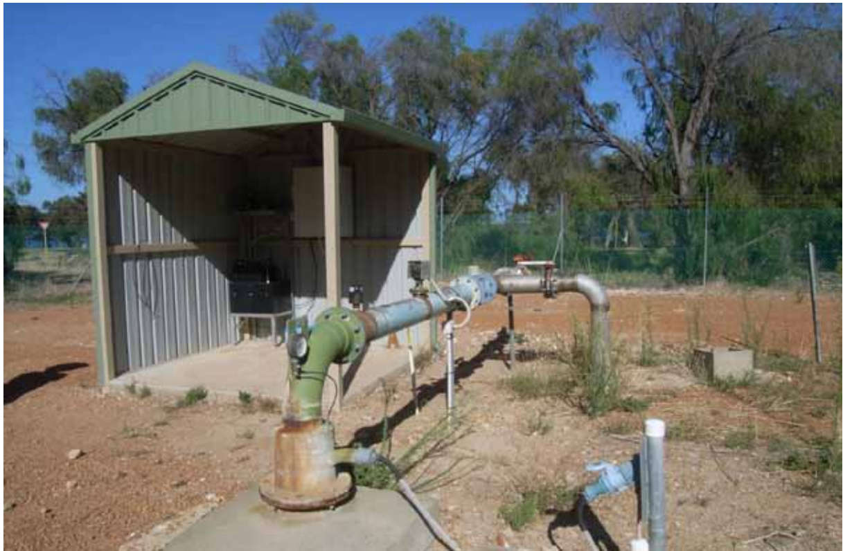
Figure C1 Australind Water Reserve production bore 1/77
