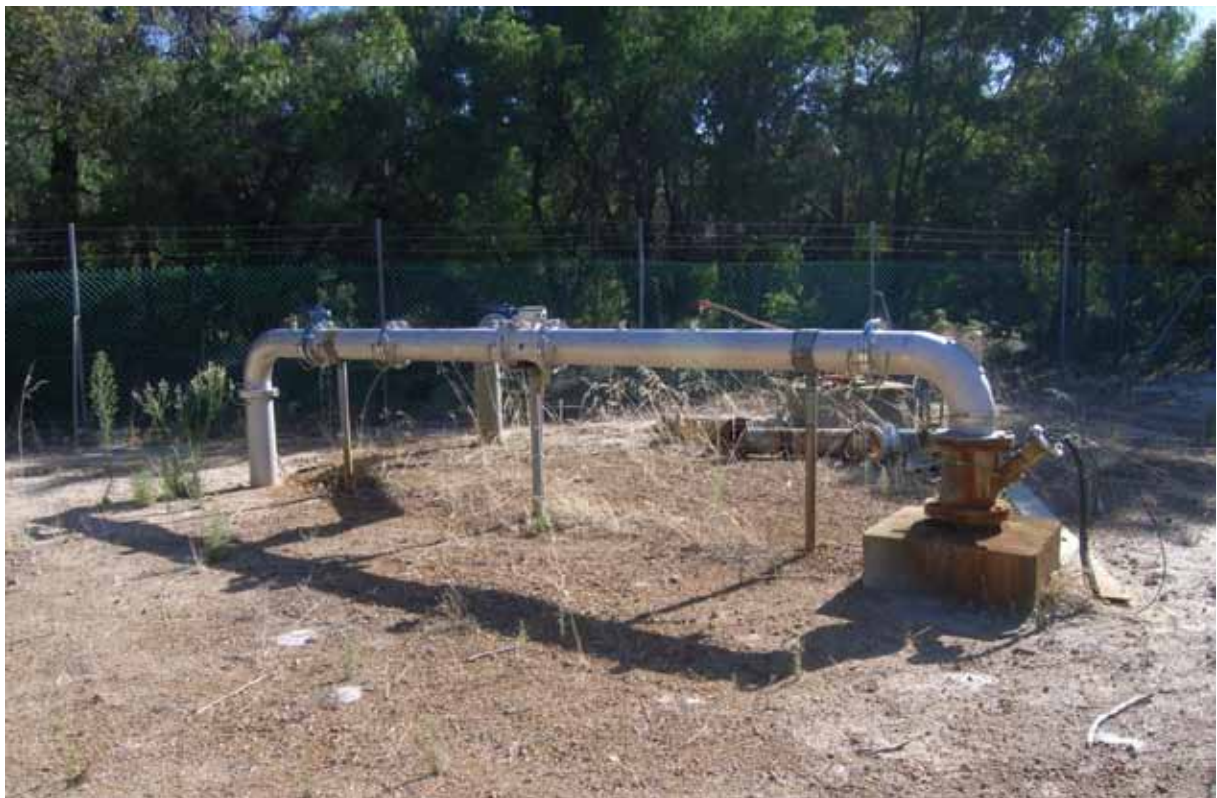
Figure C2 Australind Water Reserve production bore 1/97
