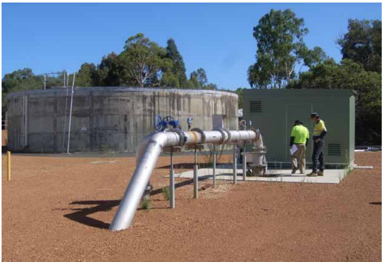
Figure C4 Australind Water Reserve production bore 1/06
