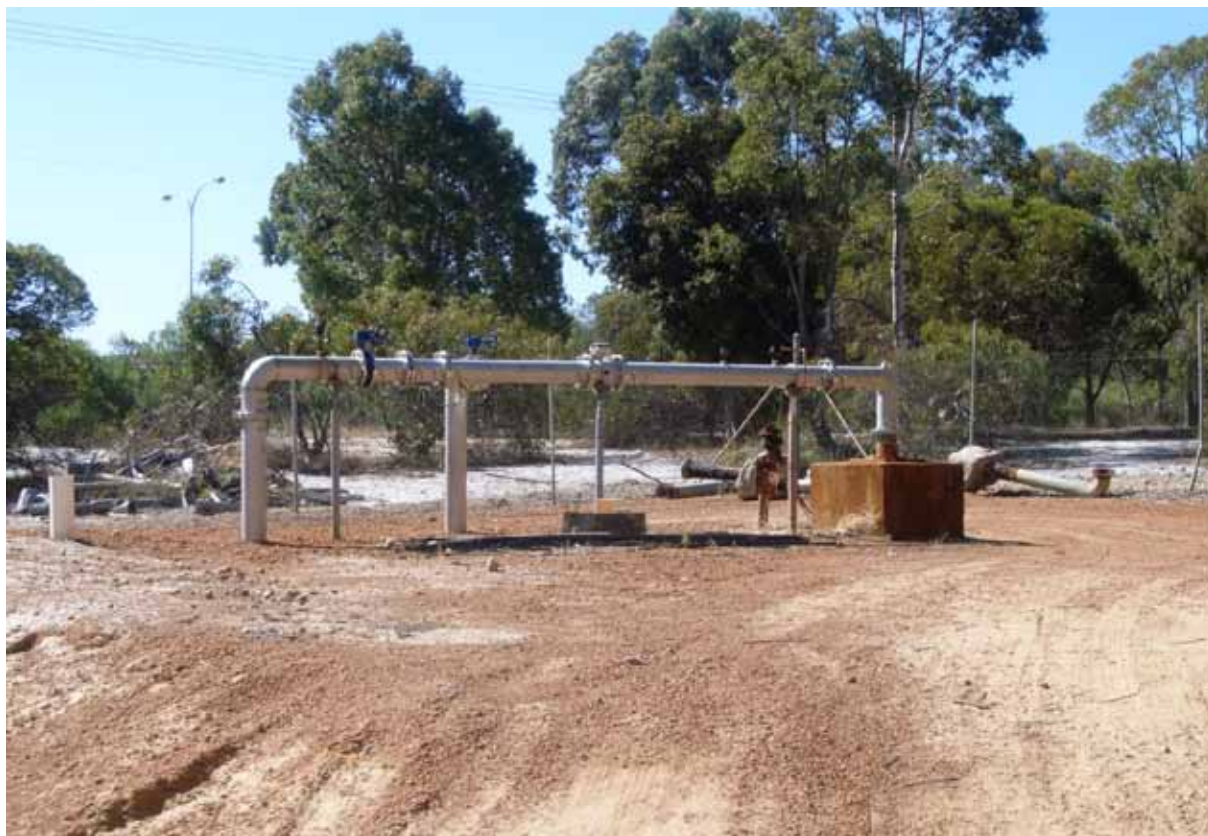
Figure C5 Australind Water Reserve production bore 1/82
