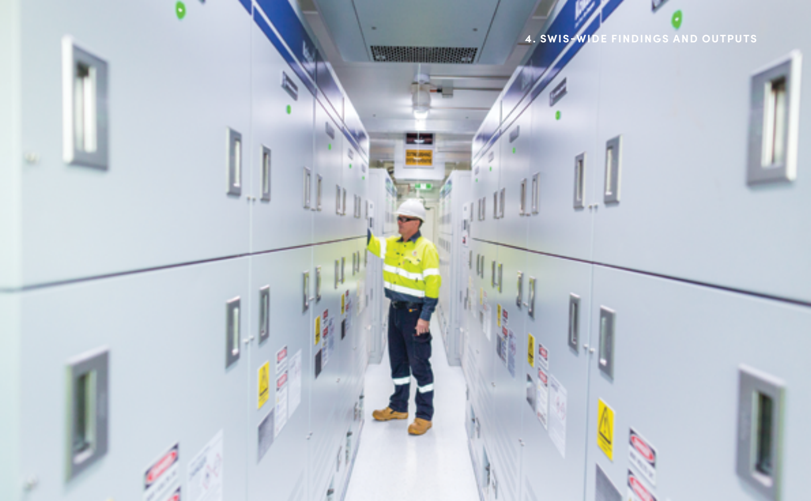
Large-scale battery storage. Source: Alinta Energy.
