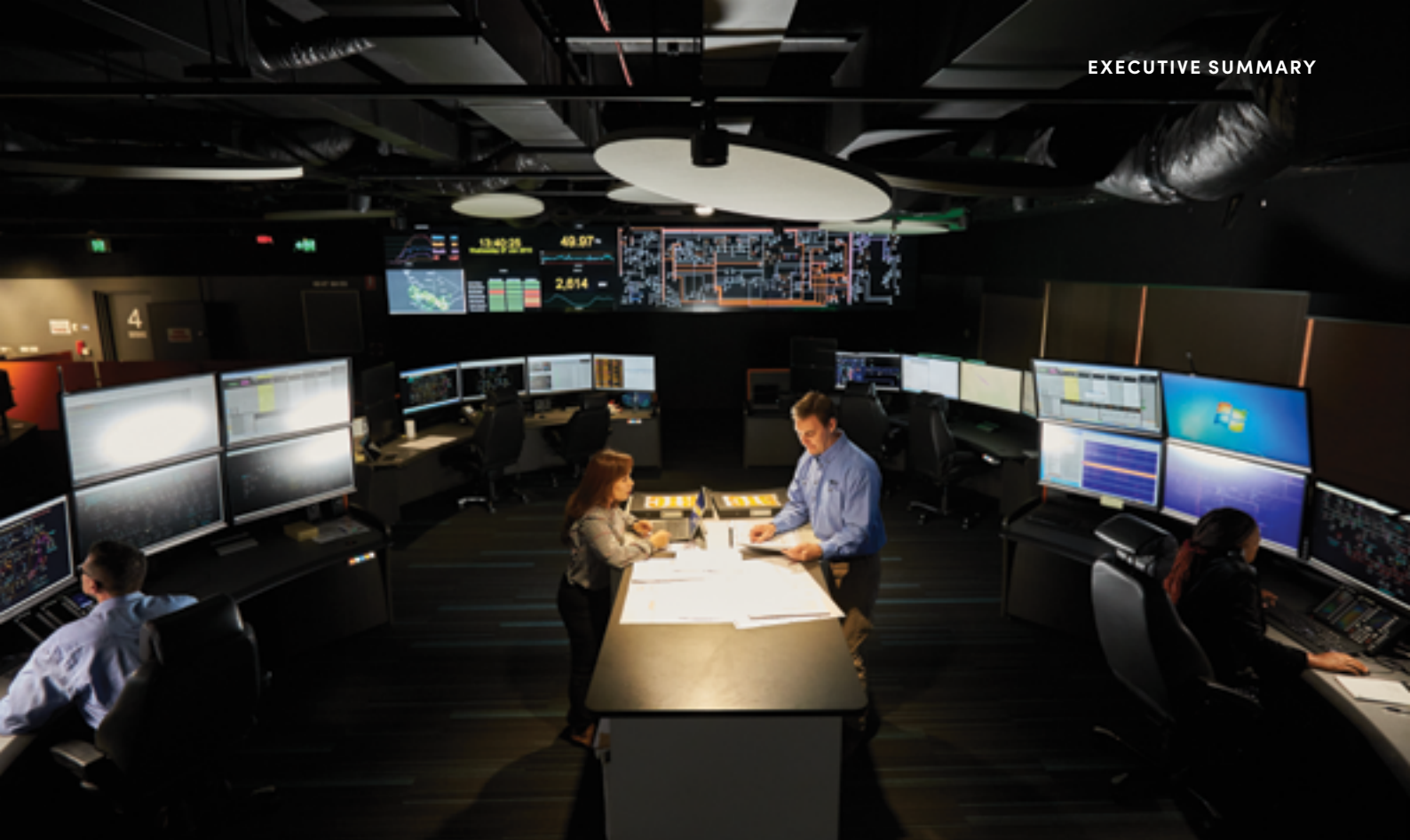
Western Power Control Centre. Source: Western Power.
