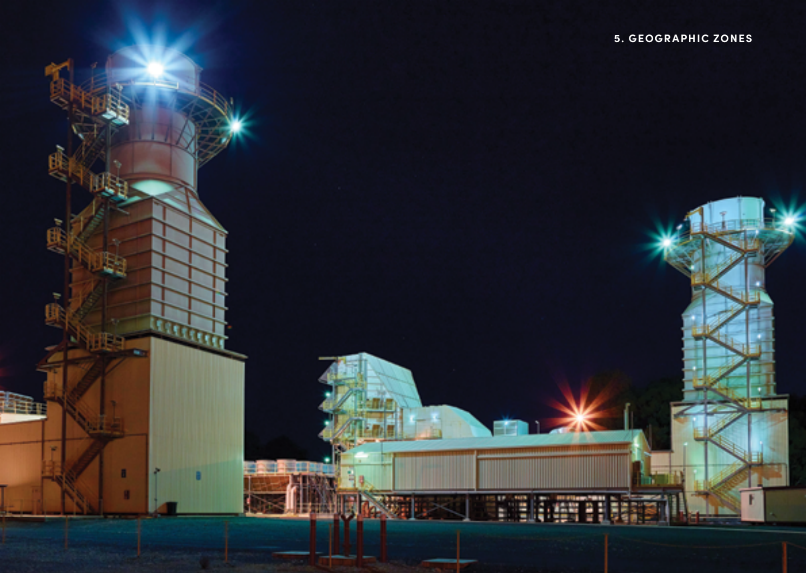
Alinta Wagerup Gas Turbine. Source: Alinta Energy.
